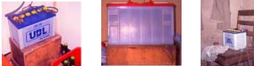
Figure 9: Examples of poor battery locations. Two batteries are placed on top of a too small battery box (left and middle). One is in a kitchen (middle), and the other two in bedrooms (left and right). (Photos from field study)
